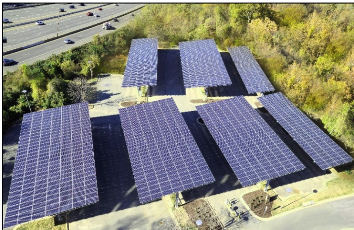
Photo 2: Solar PV Panels installed on the parking lot at The Tower Building, photo credit to Prospect Solar
