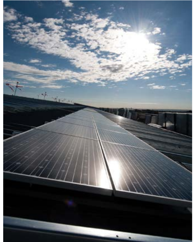
Credit: Dennis Schroeder / NREL
