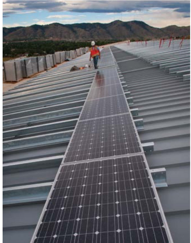
Credit: Dennis Schroeder / NREL
