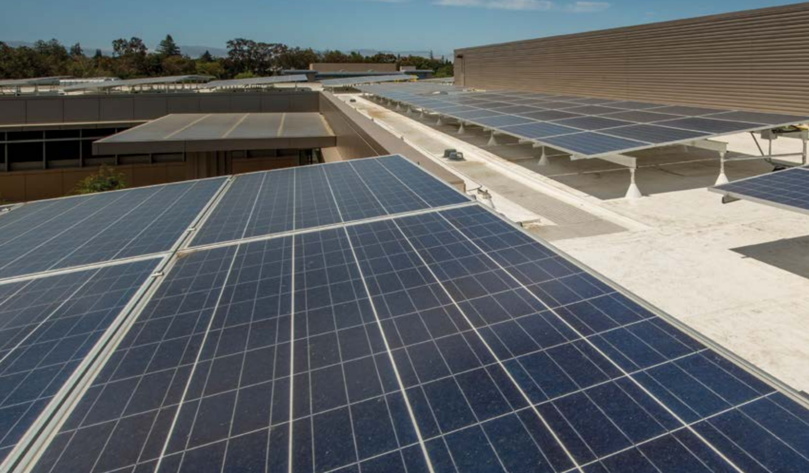
Solar panels on the roof of net zero energy Hanover Page Mill office building in Palo Alto, CA.
